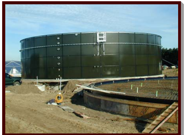
Sludge Storage Tanks
