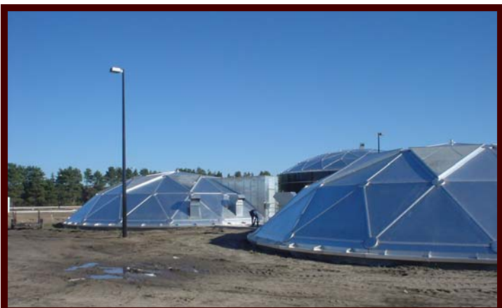
Dome Covers over Final Clarifiers
