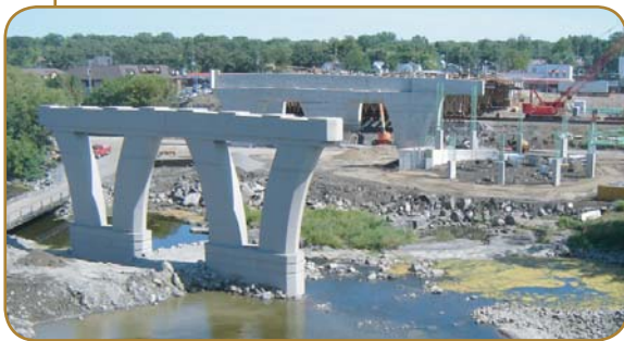
Crews worked literally around the clock during the winter of 2005-2006 to keep pier construction on schedule.
