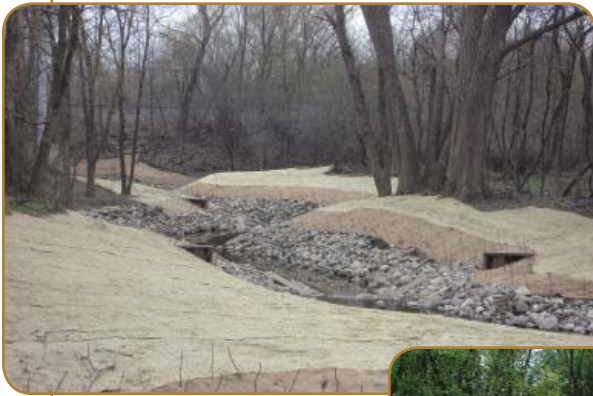
The resorted channel was covered with erosion control blankets, seed, and plantings.
